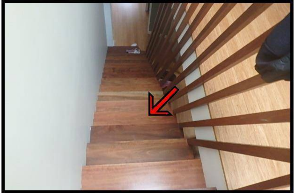
The stairs are constructed primarily from timber. The overall condition of the stairs is good.
