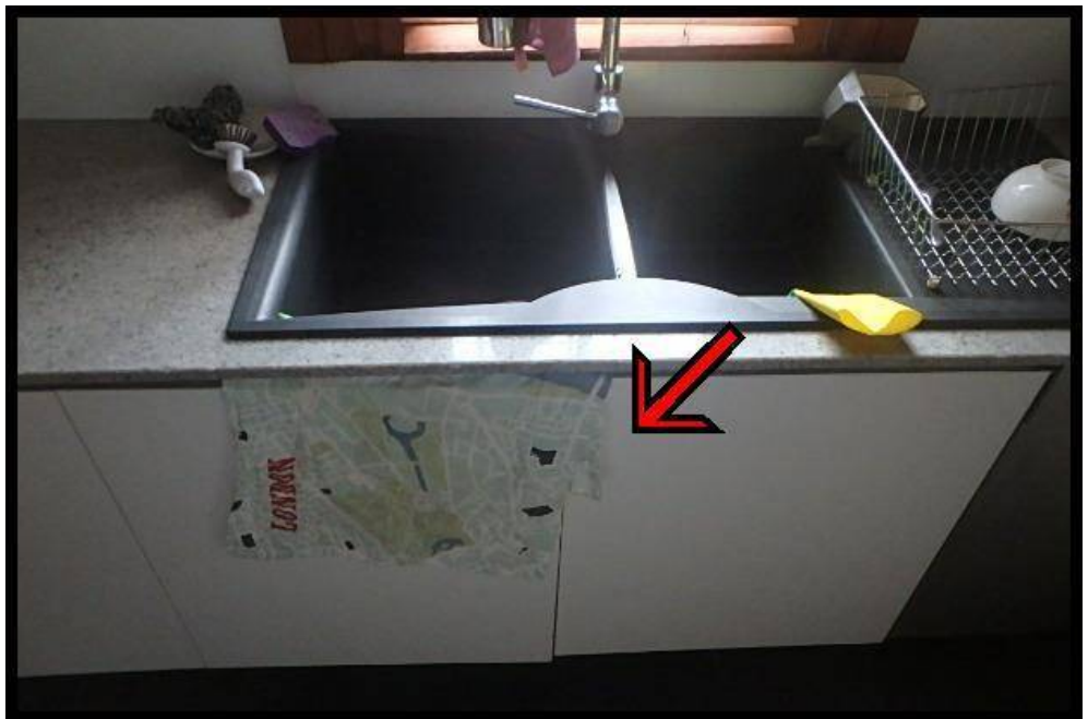
The condition of the fixtures is generally good. Adjustment is required to some door and drawers to ensure smooth operation.
