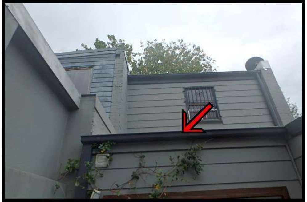
Leaves and debris are present in gutters. These should be cleared.
