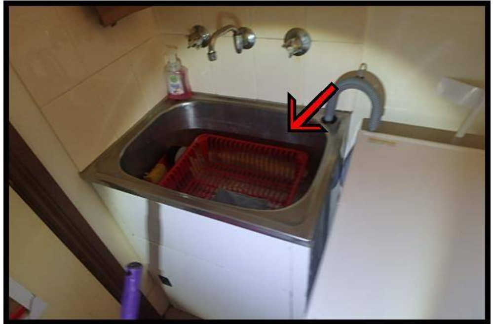
The tub and taps appear serviceable.
